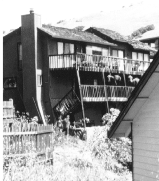
Figure 22 - This hillside home was built on an unbraced tall wall that failed.
